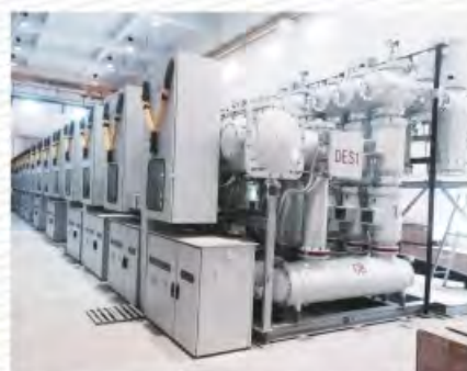
India TANTRANSCO Guindy 230 110kV GIS Substation Project
