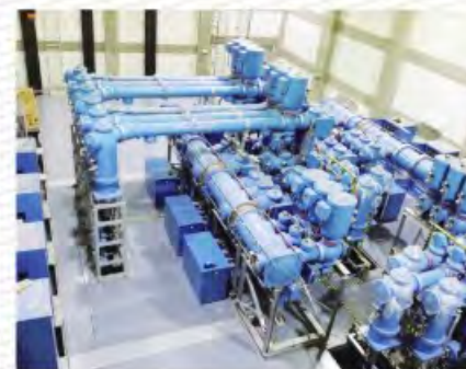
Mexico CFE 237LT 1313 252kV GIS Substation
