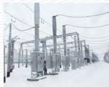
Belarus 330kV Substation Project
