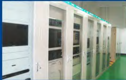
SHR5000 Substation Automation System Running in Hunan Electric Power Company
