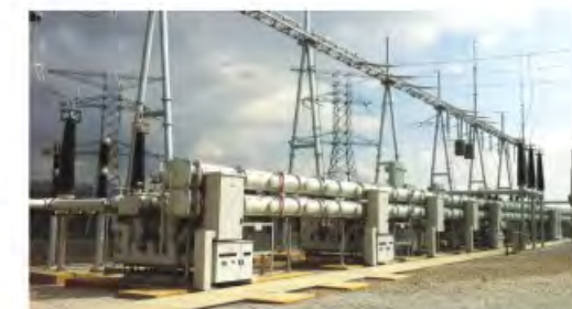
220kV Yun Nan-Jinzhong GIS Substation
