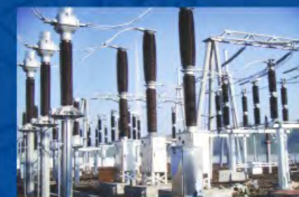
220kV Shihezi Oasis Substation
