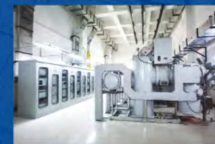
Bewu Village 145kV GIS Substation
