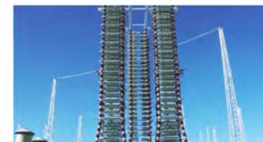
ShanghaiMiao-LinYi ± 800kV HVDC Transmission Project
