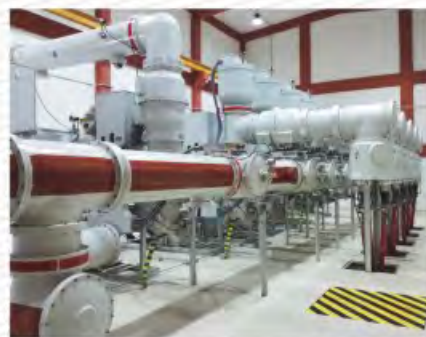
Mexico CFE 1521 115kV GIS Substation
