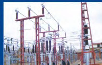
LW36-72.5 SF6 Circuit Breaker Running in Madagascar
