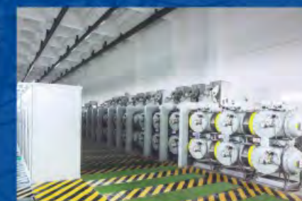
Beijing Future City Station 145kV GIS Substation
