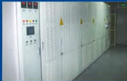
STATCOM Running at Shanghai Expo Mengzi Substation
