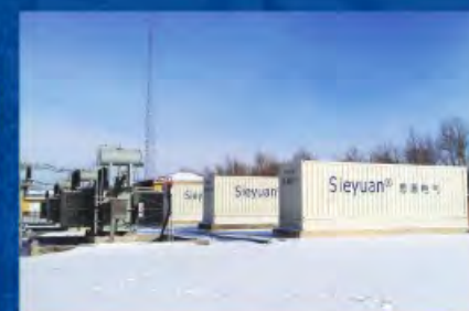
33kV STATCOM Project in Jilin Wind Farm
